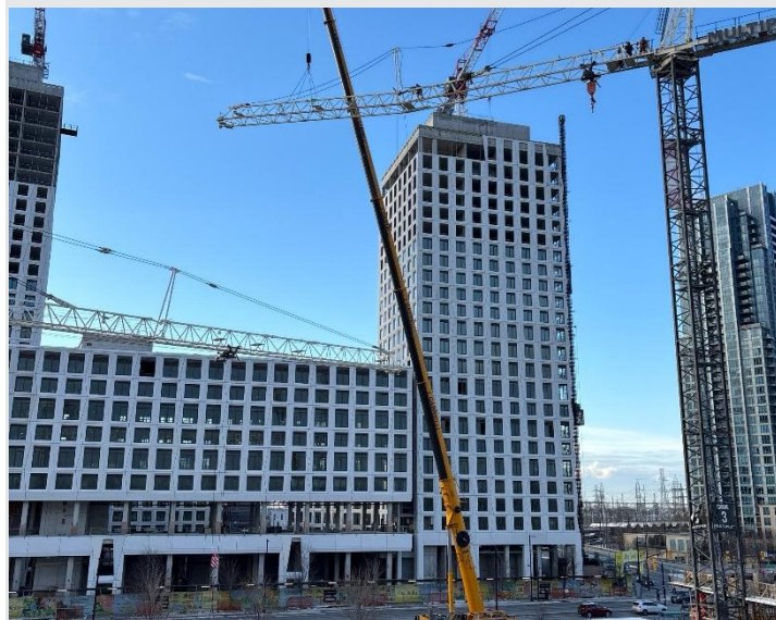
Pictured: Changing The New Etobicoke Civic Centre's Tower Crane #3 from a "Hammerhead" to a "Luffer".
