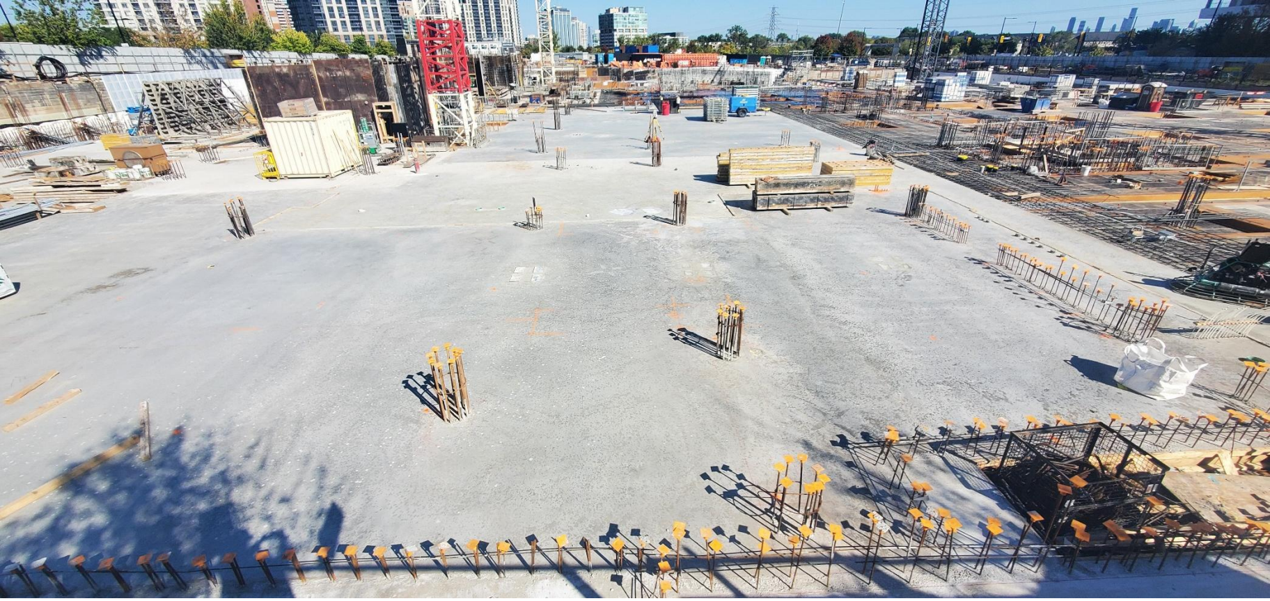
Pictured: The New Etobicoke Civic Centre progress update as of October 2025 - Level 00 (Ground Floor) Concrete Slab
