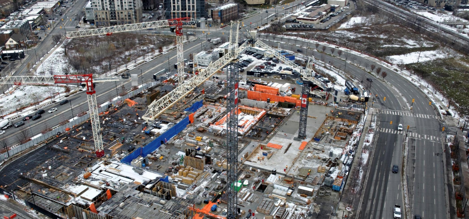
Pictured: The New Etobicoke Civic Centre progress update as of December 2025 – Aerial Site Overview
