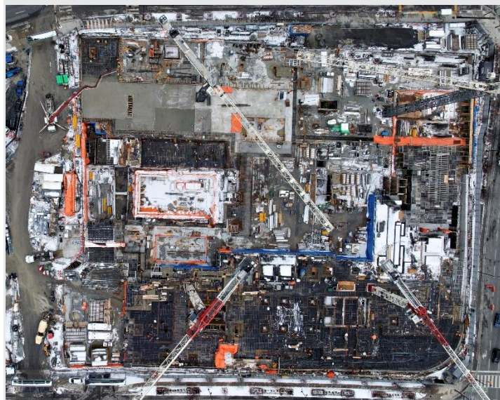
Pictured: A top-down view of the concrete decking progress on Level 00 and 01.
